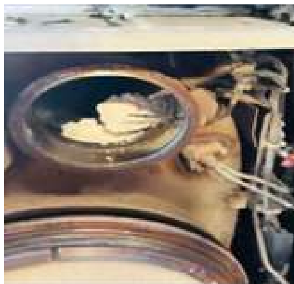
Figure 1. Solid deposits observed during inspection of an SCR system
