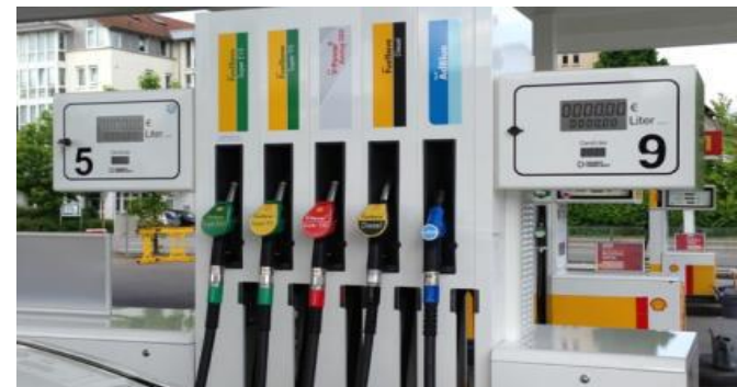
Dispensing units at fuel retail outlets
