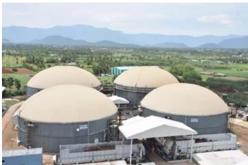
200 TPD Plant at Namakkal, TN By IndianOil-Adani Venture
